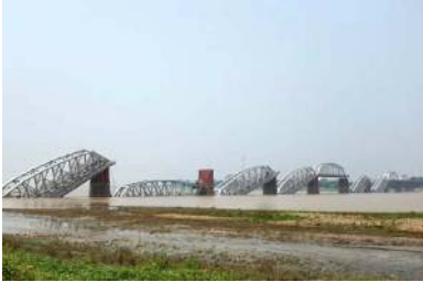
The collapsed Ava Bridge in Mandalay [EPA]
